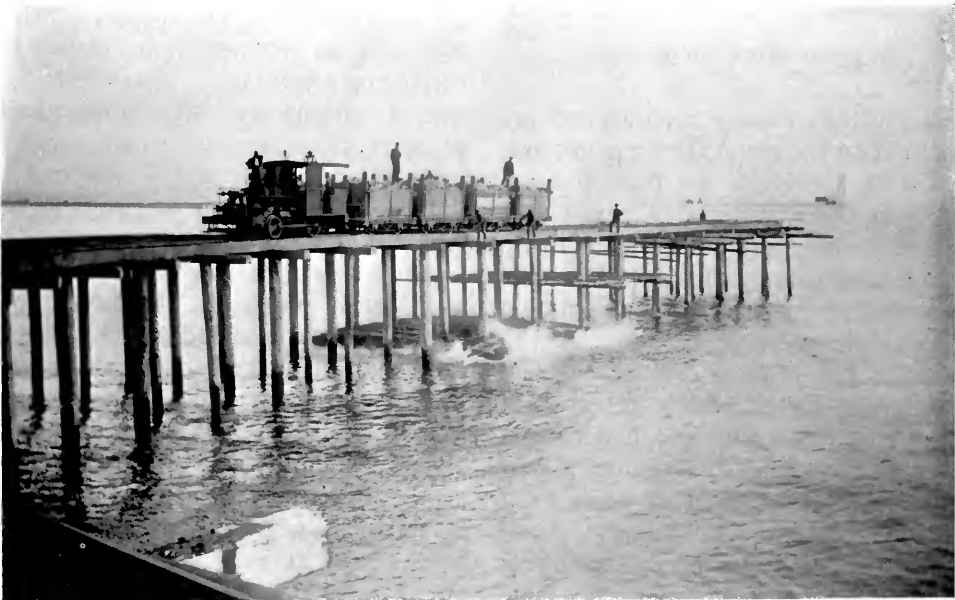
WITH A CRACKLING SOUND THE MATTRASS STRIKES THE WATER.
